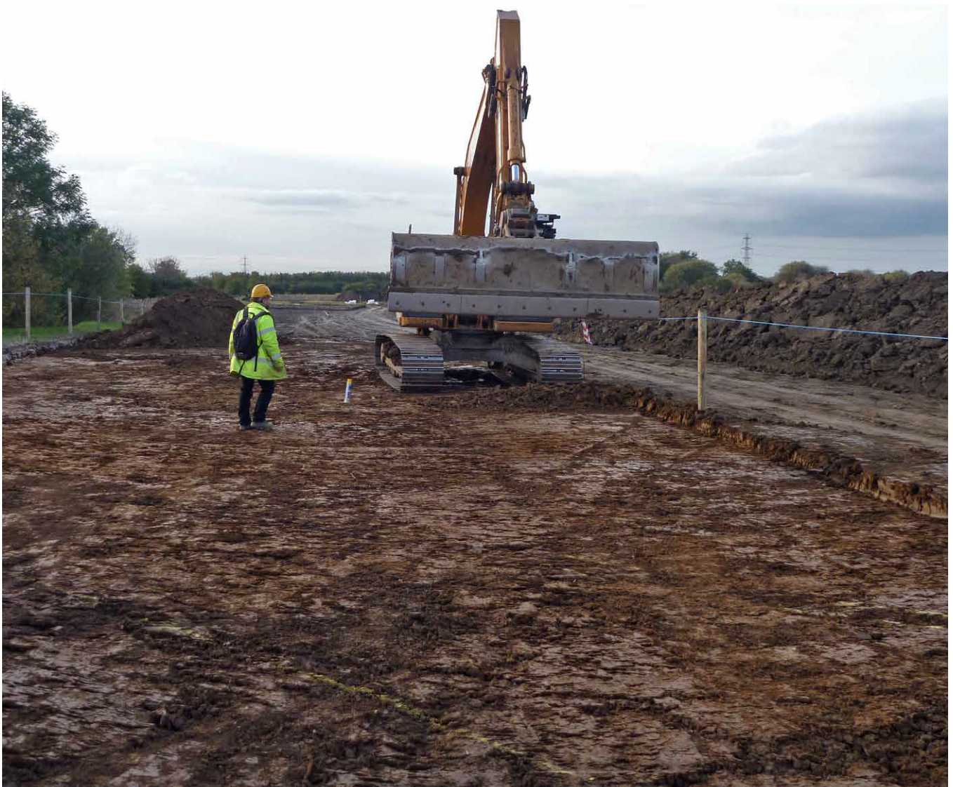
Figure 5 Construction vehicle load and rutting from wheels can cause damage to archaeological deposits.
